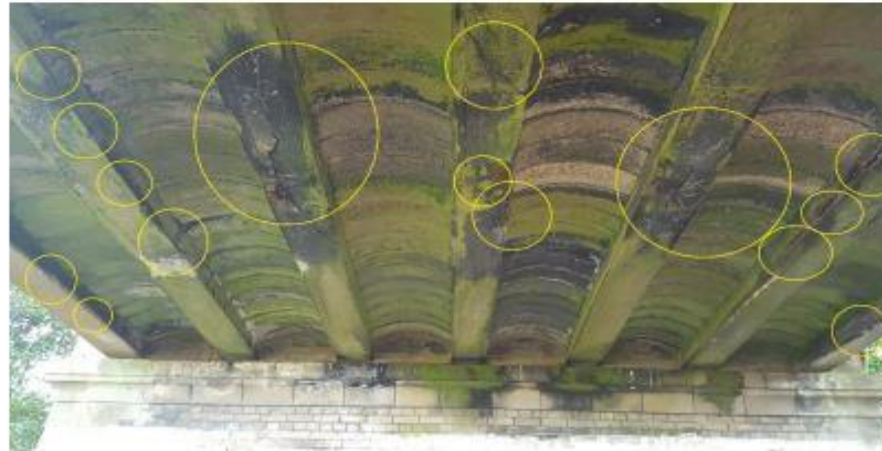
Concrete encasement around each beam had also fractured (highlighted) and spalled.
