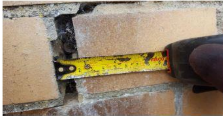
Close up photo of fracture in north side abutment, fracture measuring 25mm.
